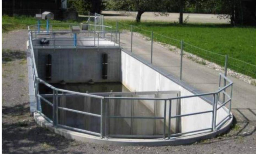
Figure 6.18 Units based on filtration: A pre-sedimentation catchbasin (in front) and a down-flow media filter treating first flush (15 min, one-year return period) in Austria (Photo: Courtesy of ASFINAG).
