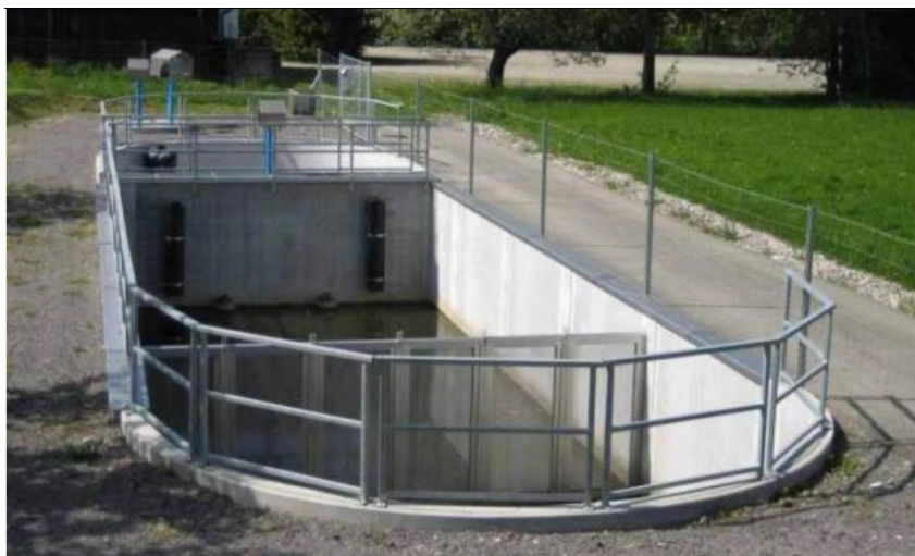
Figure 6.18 Units based on filtration: A pre-sedimentation catchbasin (in front) and a down-flow media filter treating first flush (15 min, one-year return period) in Austria (Photo: Courtesy of ASFINAG).
