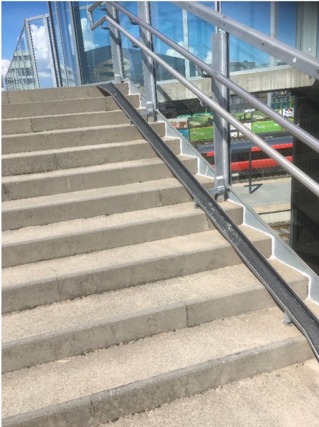
Fig. 4. Illustrative example of a stair roll track for bicycles. Source: Svein Johan Knapskog.
